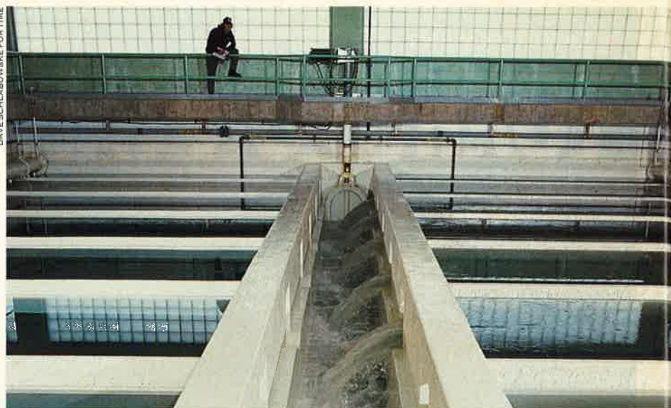
Laid low by a nasty microorganism last spring, Milwaukee promptly spent $1 million to upgrade treatment plants like this one, which filters water through sand
